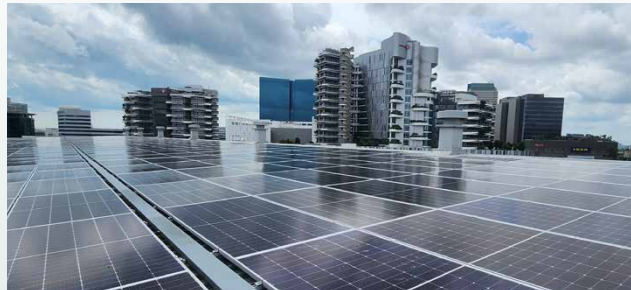
Tapping on renewable energy with solar panels installed on the rooftop of IMM Building
