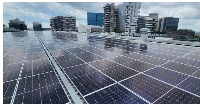
Phase 1 installation of solar panels at IMM Building
