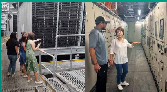
From left: Site inspection of access platforms and safety railings checks at Capital Tower.
